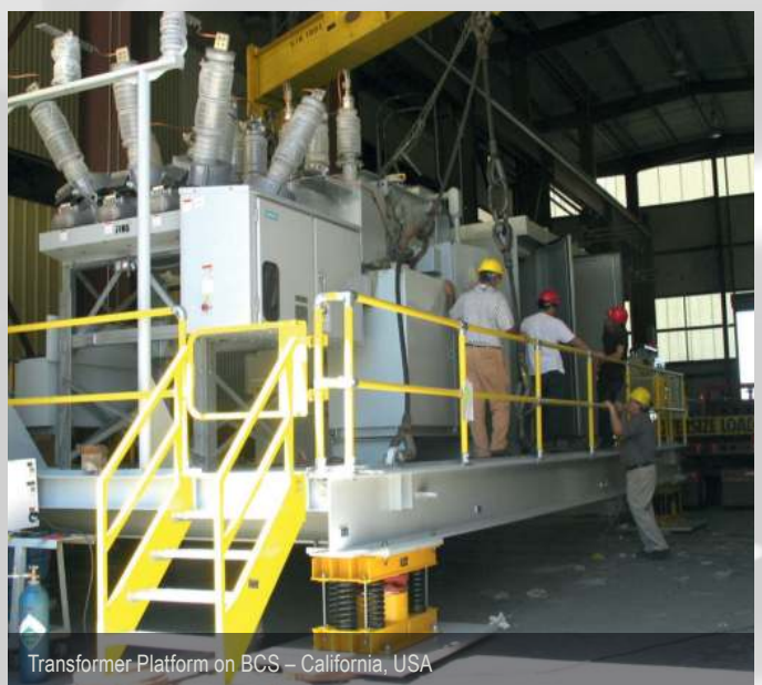
High Voltage Reactors with Earthquake Protection – California, USA
